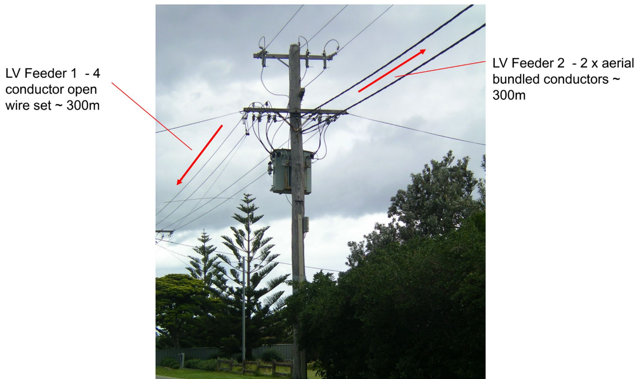
Figure 7 – Typical LV Network that will Require Major Augmentation/Rebuild under the Step Change Scenario (2050)
